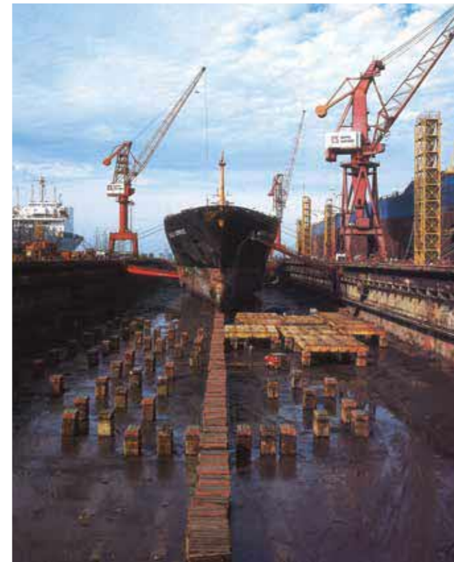
A ship undergoing repair in Keppel Shipyard, c. early 1990s. Image reproduced from Lim, R. (1993). Tough Men, Bold Visions: The Story of Keppel (p. 65). Singapore: Keppel Corporation Limited. (Call no.: RSING 338.76238309 LIM).
